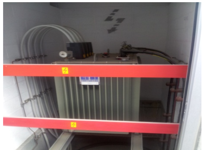
FIGURE 5. Transformer deployed in the Techno-pole.
