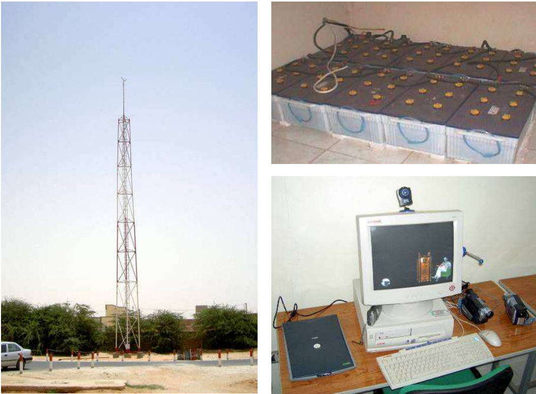
Figure 1: Antenna for the Internet connection, Backup energy source and e-learning and teleconsultation equipment
